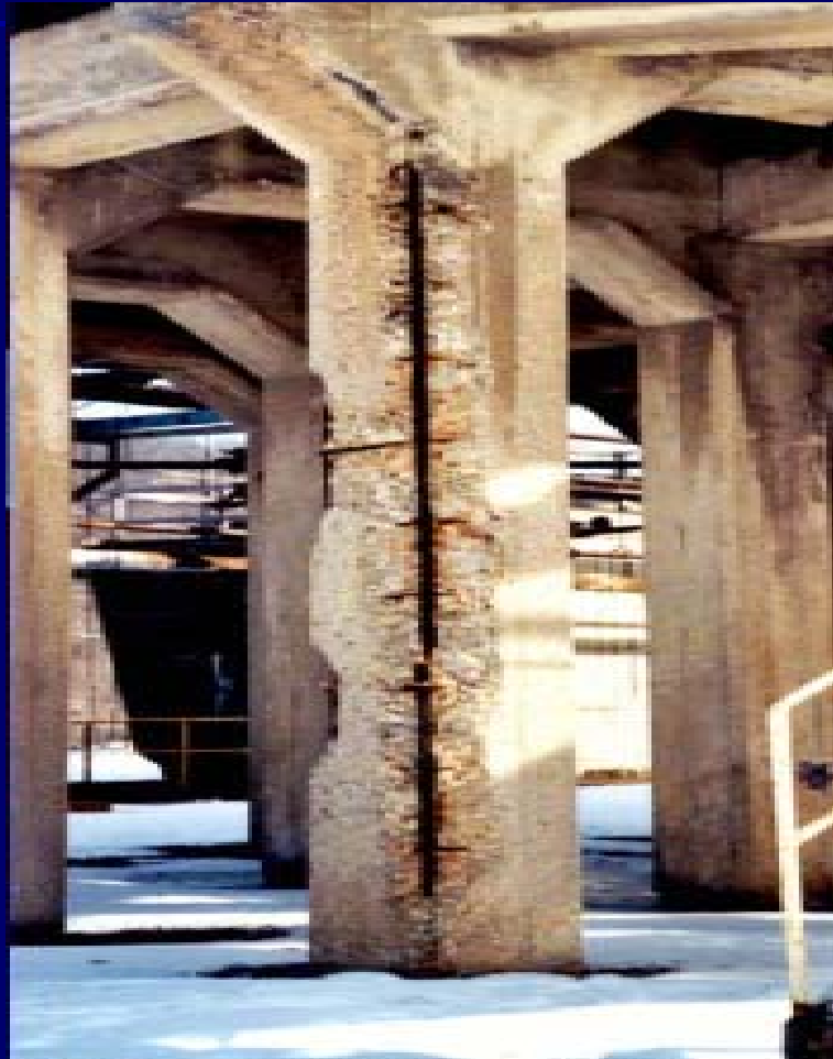
Concrete spalling by rebar corrosion in column
